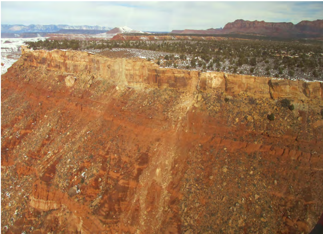
Figure 9. Upper part of the path taken by the December 12, 2013, rock fall. Note how pre-existing small gullies on the Moenkopi slope split and redirected a portion of the rock fall. Numerous freshly fallen boulders of unknown stability remain on the slope along the rock-fall path. Photograph taken on December 13, 2013, view is to the northwest.
