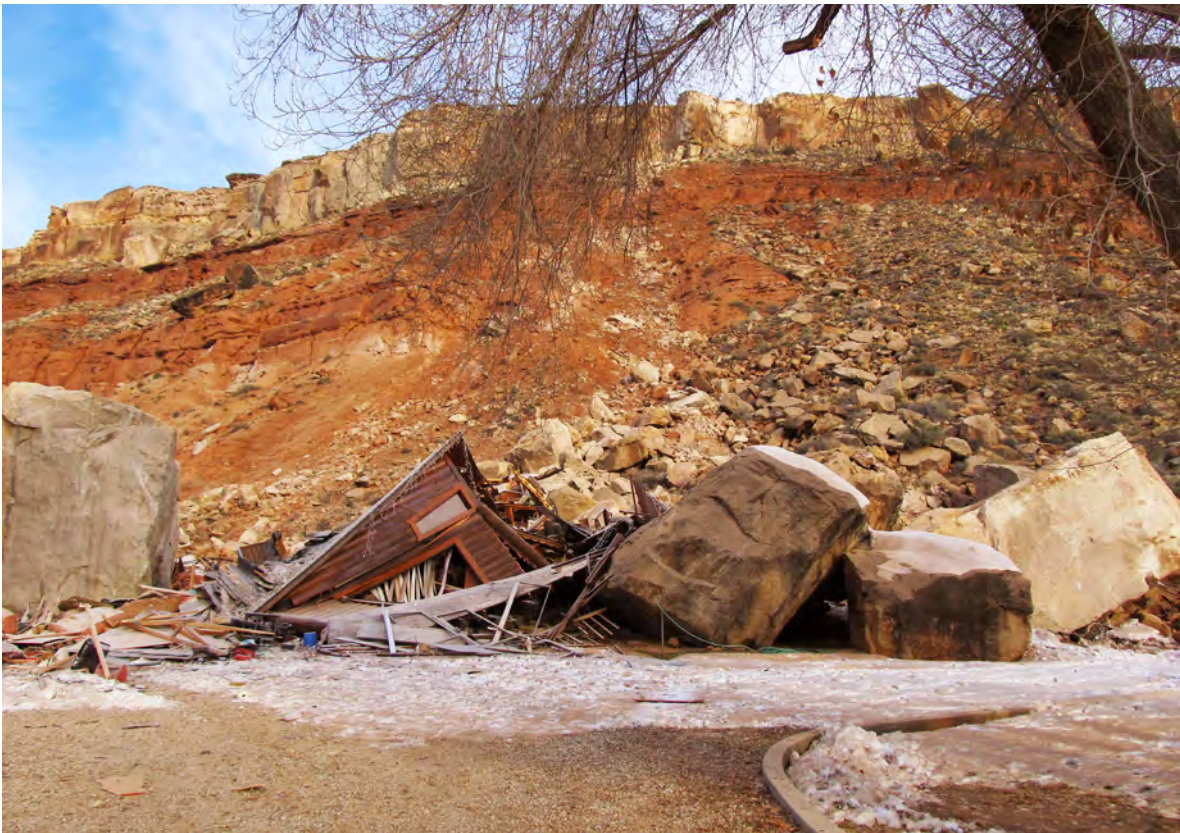
Figure 3. Remains of the house at 368 West Main Street, Rockville, Utah, following the December 12, 2013, rock fall. Photograph taken December 13, 2013, view is to the north.
